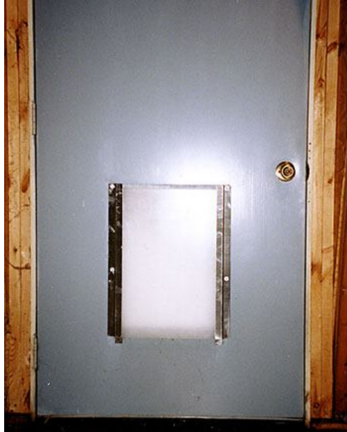
An installed closure on metal door Photo 2
