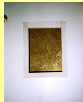
Frame the inside and outside of the hole on the door – use 1/4" cedar or pine 2" wide.
