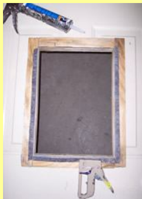
Use silicone caulking around trim kit for add insulation. To quiet door closing staple 5/8" window felt to sides and bottom.
